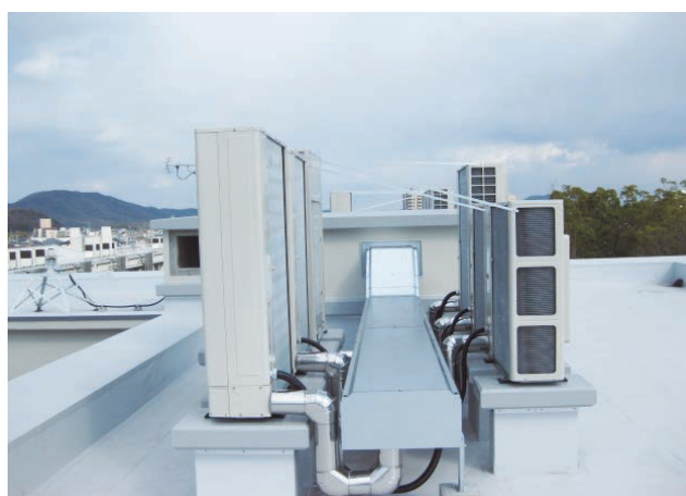
Faculty of Education Lecture Hall Rooftop (High-efficiency air conditioner/ Rooftop heat insulating and waterproof materials)
